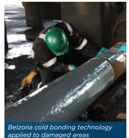
Corroded area and leaking hole on the methane pipework
