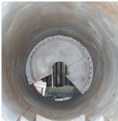
Thin-wall defects on mixer
