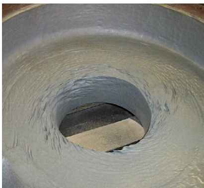
Entrainment damage on slurry pump
