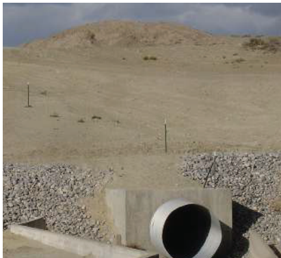
Pipe used to carry irrigation water
