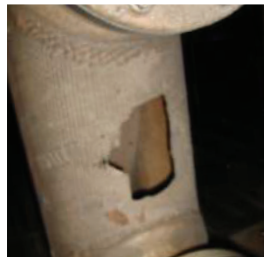
Damage to pipework
