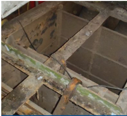
Eroded rubber lined tanks
