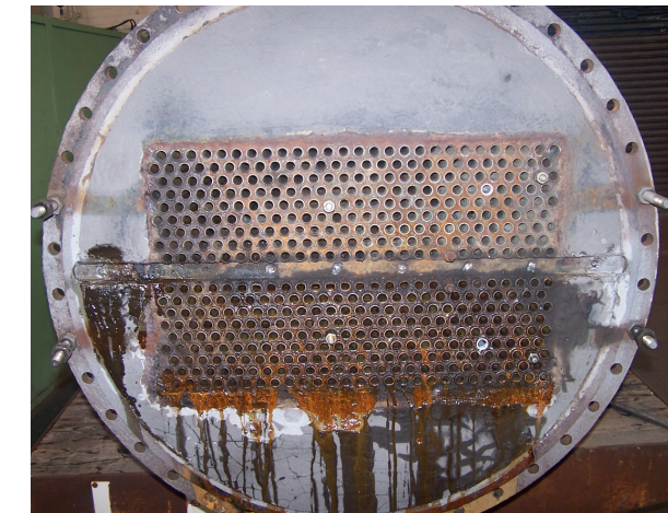
Deterioration of previous linings
