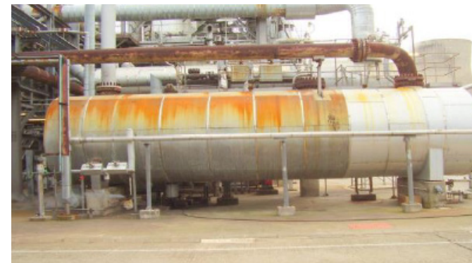
A vessel operating at high temperature experiencing corrosion and wall thinning in service.
