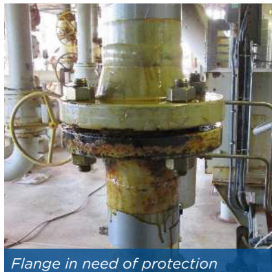
Flange in need of protection
