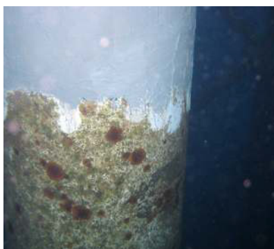
Corroded platform leg
