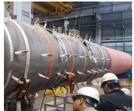
Riser bearing bonding
