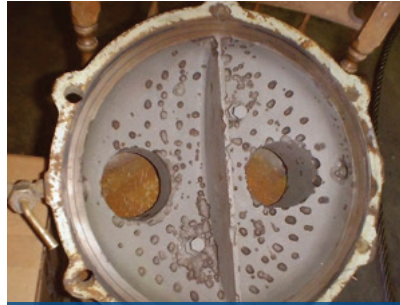
Severe pitting on division bar
