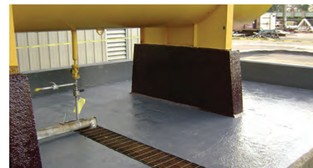
Sulfuric acid containment area coated and protected
