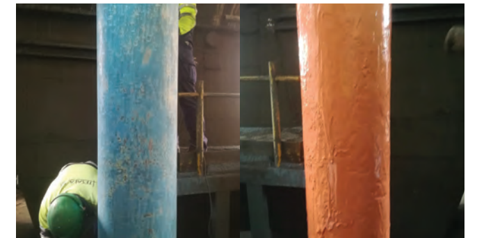
Exposed hot pipeline made safe with insulation
