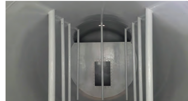
Internal coating for high temperature tank
