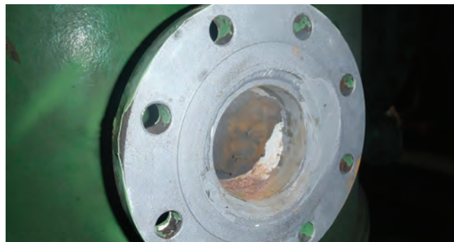
Flange face after grit blasting and deep pitting
