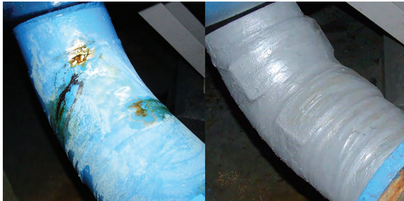
Internal corrosion resulting in pin hole leaks
