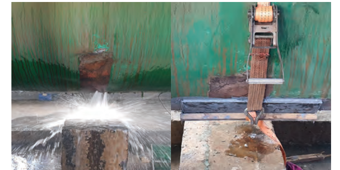
Live leak on a pipe sealed with Belzona
