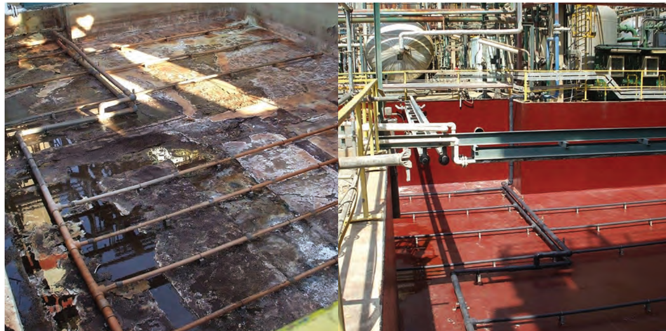
Severe damage to the coating and concrete from chemicals
