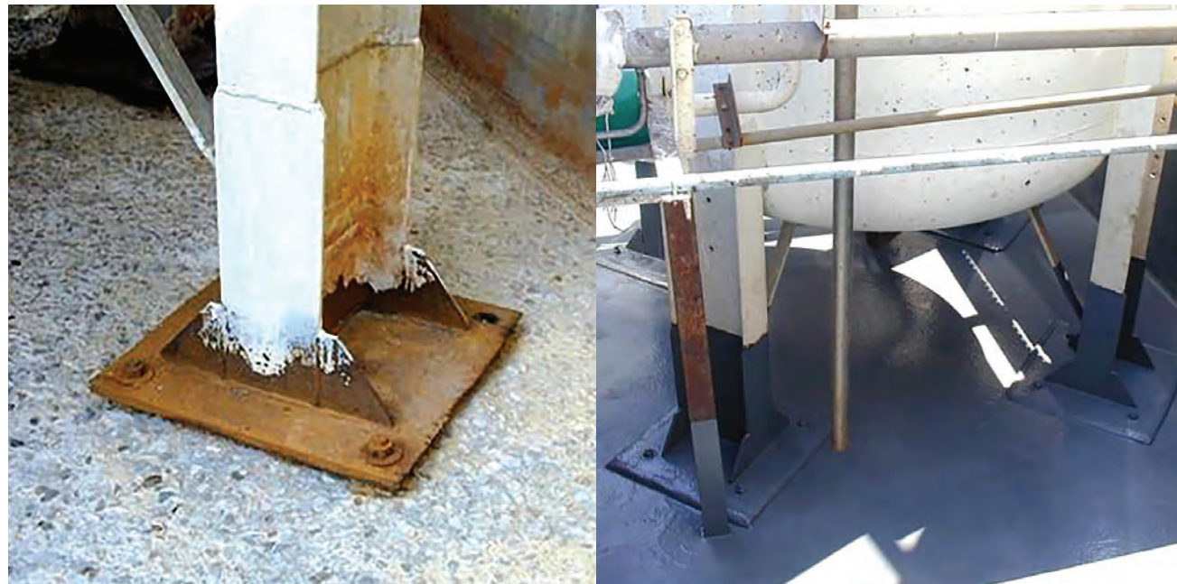
Deterioration of the concrete due to leakage and contamination Shimming and protecting base of support steelwork
