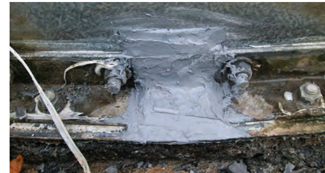
Tank base causing local flooding sealed
