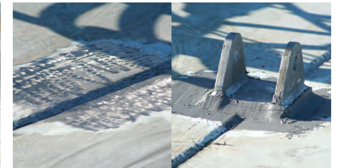
Plates bonded on top of a water tower for radio dishes
