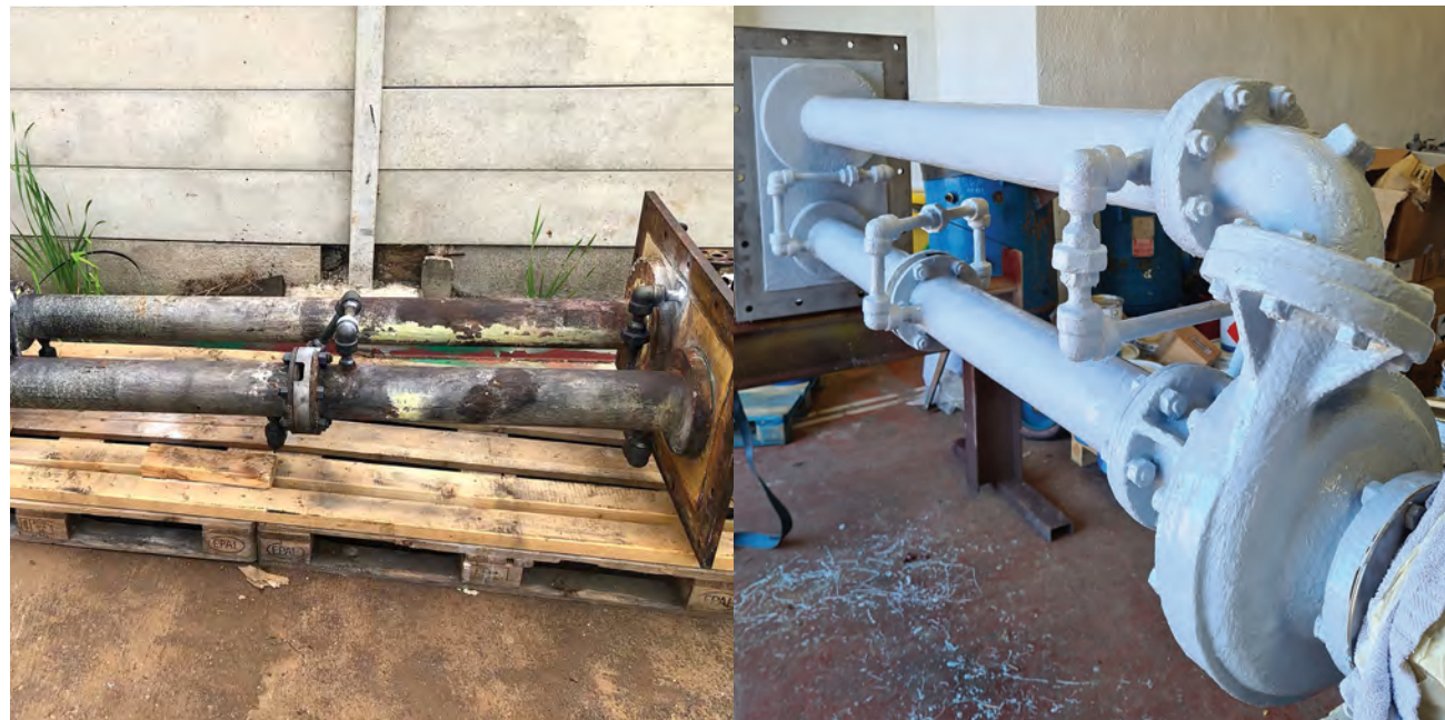
Short working life of pumps due to high corrosion
