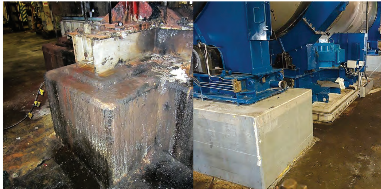
Damaged concrete plinths
