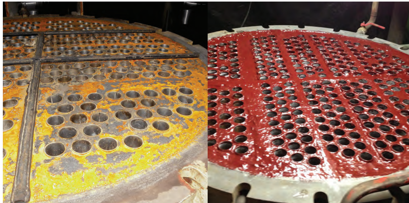
Degradation of surface due to high temperature acidic media
