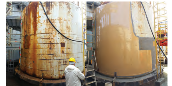
External corrosion protection on tank
