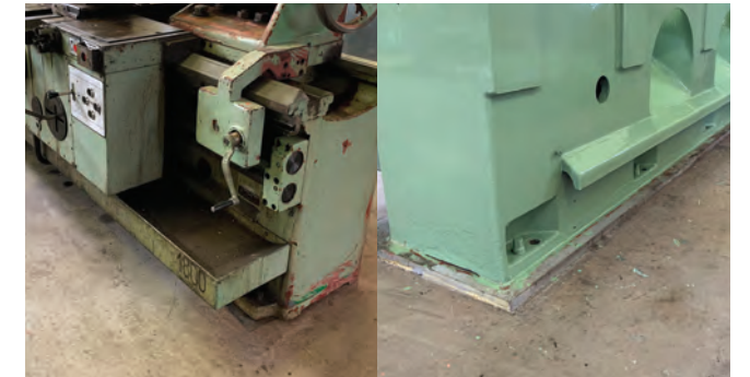
Installed lathe required chocking for stabilization
