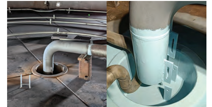
Storage tank protected against high temperatures
