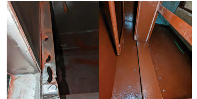
Scrubber vessels coated to protect from chemical attack
